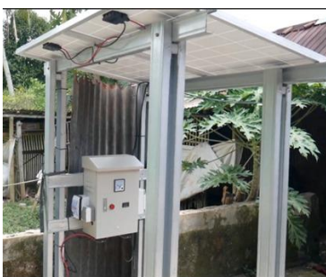
Gambar 4. Instalasi Panel Surya
